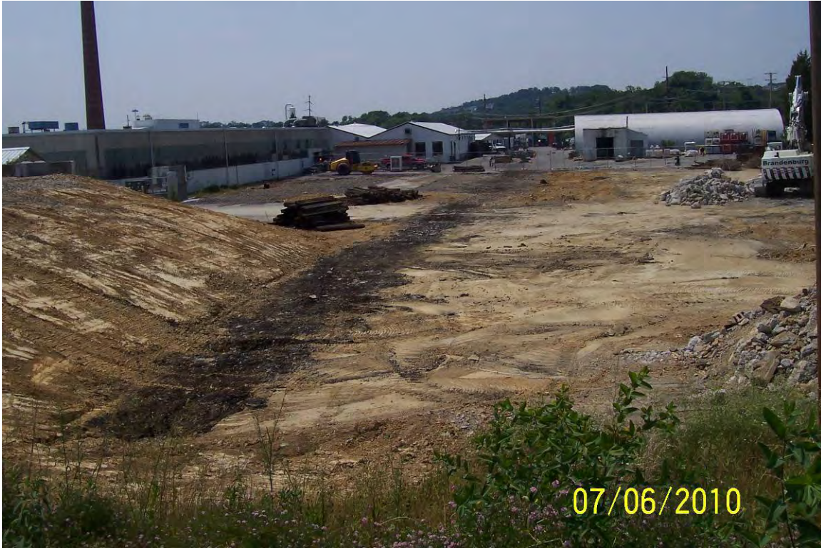
Views looking west from east side of new sedimentation pond (#3). Note pre-excitation conditions – Concrete walls, bins and platform have been removed from MCB. Dark area is former railroad – ties and rails removed.
