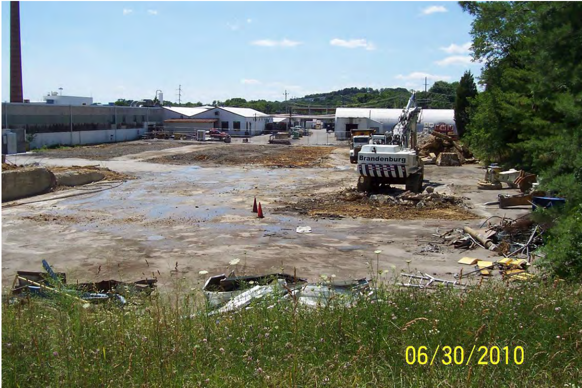
View looking west at demolition areas for Bldgs 12, 43, 44, & 67 (Bldgs 42, 57 & 51 in background). Trackhoe is sitting on former Bldg 67.
