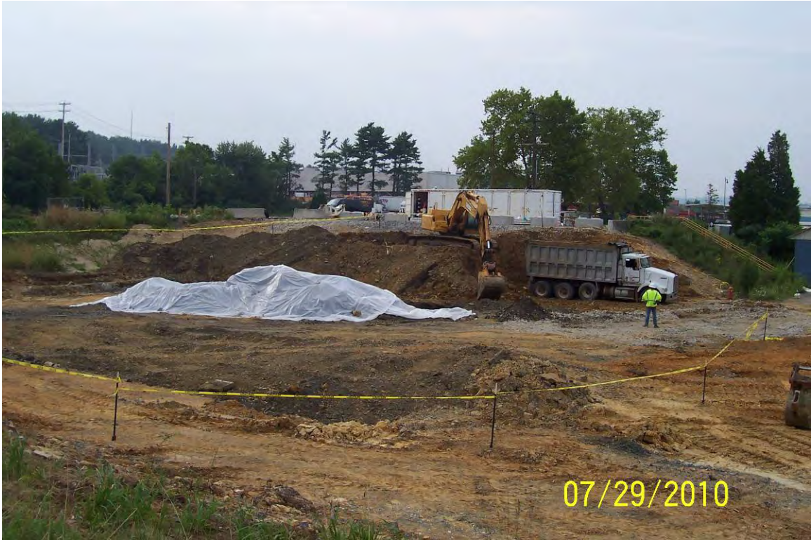
View looking southeast at excavation along hillside of former MCB area. Soil above contaminated zone was removed, stockpiled near Bldg 15 (below) and tested.
