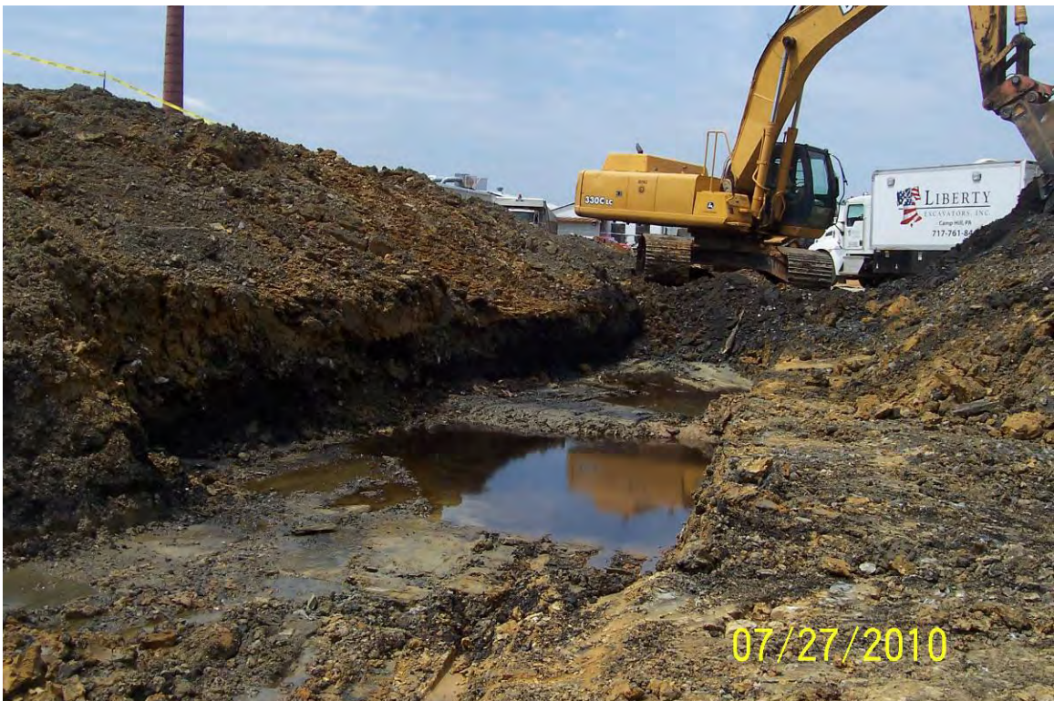
Views looking west along former railroad bed and metal chip bin area – excavation and stockpiling of contaminated soil.
