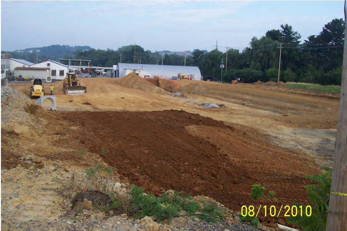
View looking west of backfilling near former MCB area and construction of new stormwater detention pond.
