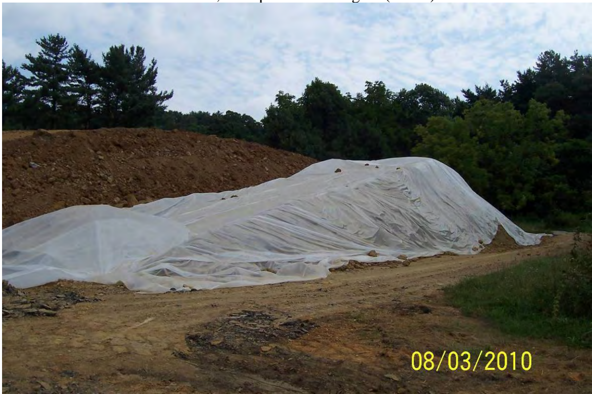
View of stockpile of suspect soil removed from the hillside of the metal chip bin area.
