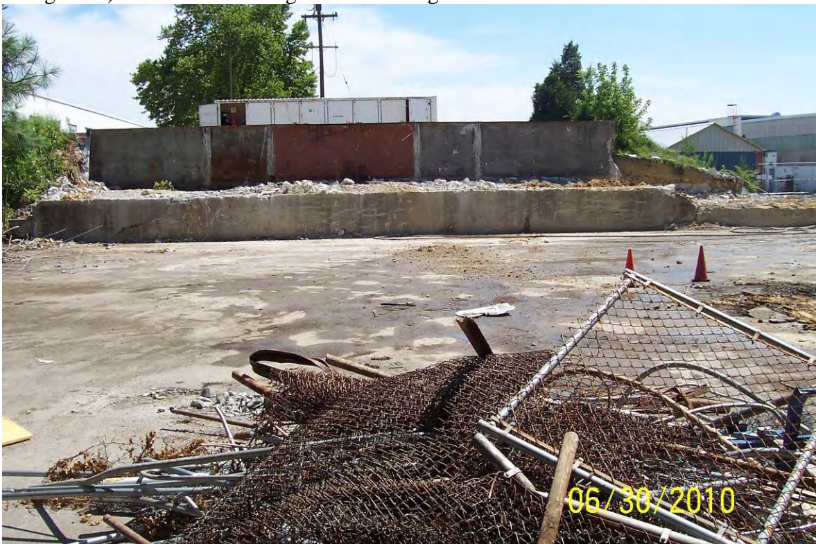
View looking south at former metal chip bin area (partially demolished). Note concrete wall next to former railroad.
