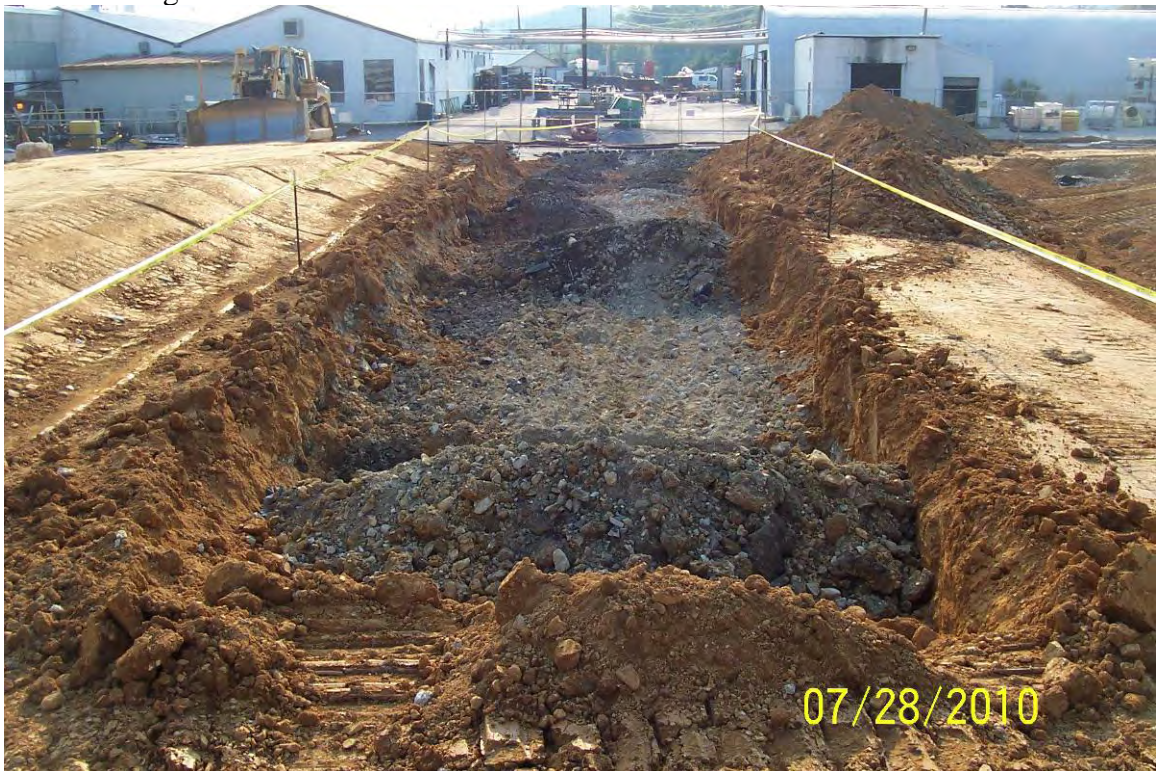
View looking west along former railroad tracks, west of MCB (beneath former Bldg 44). Note N-S oriented exploratory test pits along RR bed path.
