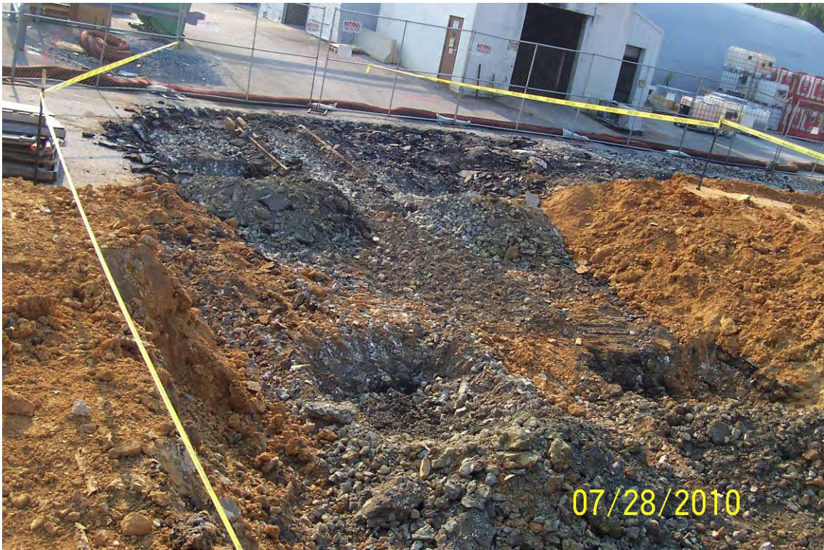
Looking west at test pits A, B, C, & D. Note location of former railroad tracks.
